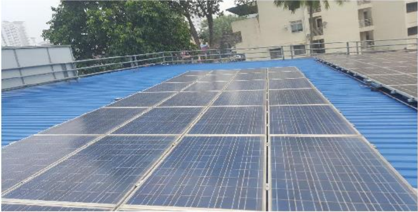
Figure 1: GCPV System Retrofitted on a Metal Roof (Source: Nor Zaini Zakaria,2018)
