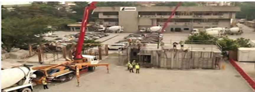
Figure 8: The trailer mounted boom truck concrete pump delivering the concrete to the constructed building (Respondent A)
