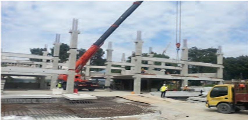
Figure 3: Mechanisation: The use of a mobile crane to lift precast components (Teraju Precast Services Sdn. Bhd., 2015)
