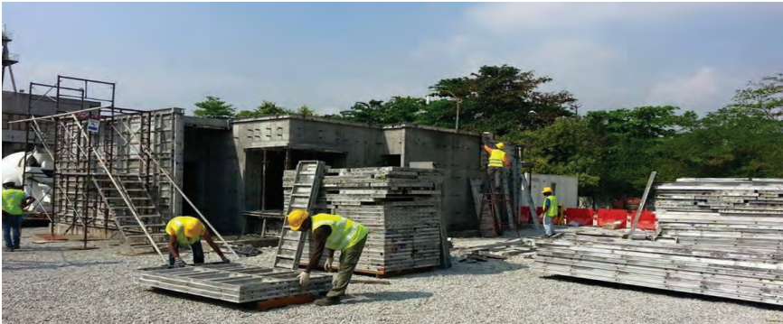
Figure 7: FASTBUILD monolithic building system using a single cast aluminium formwork system with self-levelling and self-compacting concrete (Agilia) - (Respondent A)
