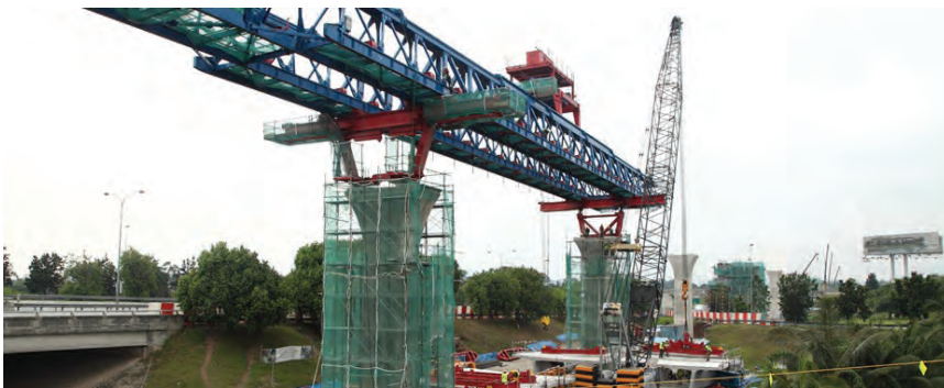
Figure 9: The MRT gantry launcher of Package V6 assembles the precast segments on the site (Respondent B)
