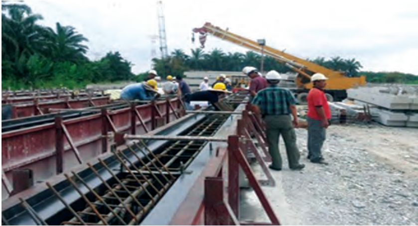
Figure 2: Prefabrication of precast beams at an off-site yard (Teraju Precast Services Sdn. Bhd., 2015)
