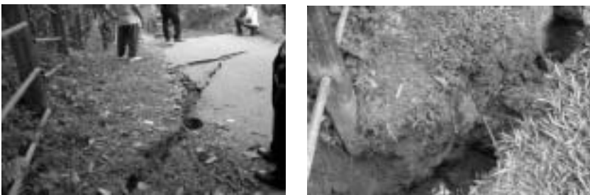
Figure 2: The development of tension crack at the crest of slope surface in which the present of rainwater will expedite the potential slope failure. Picture was taken at Wangsa Maju, Kuala Lumpur
