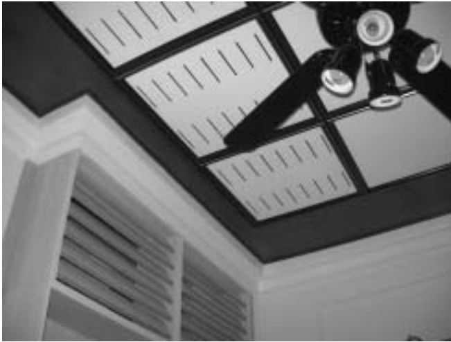
Figure 7: Internal Ventilation through the Ceiling and Wall
